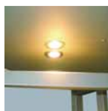
flush mounted walkway downlights
